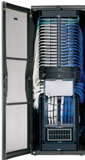
(Nexus 7010 "Heavy Copper" Pre-Configured Physical Infrastructure shown)
