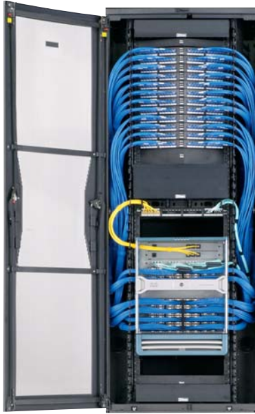
(Nexus 7009 "Heavy Copper" Pre-Configured Physical Infrastructure shown)
